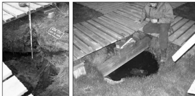
Figure 5. Sinkhole that has formed in the last couple of years within the courtyard of the Depot. The hole fills with groundwater that is warmed by exposure to surface air and then warms surrounding frozen ground. Drainage appears to be the issue. (Photos from Parks Canada and K.Skafffeld)
